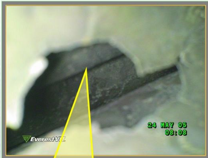
View Looking through Tube to Adjacent Tubing
