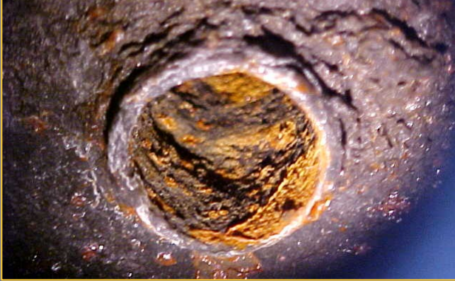
Heavy fouling and tube end corrosion
