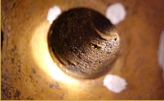
Ammonia bisulfide corrosion/pitting within roll area
