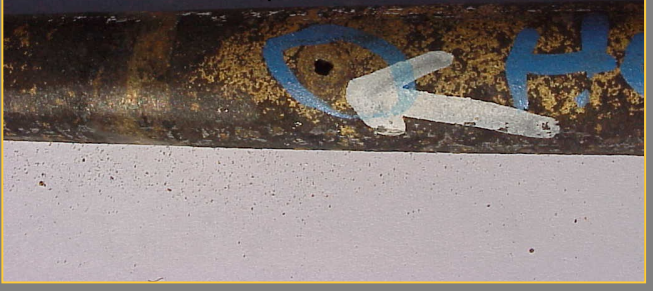
Removed Sample Tube with Failure
