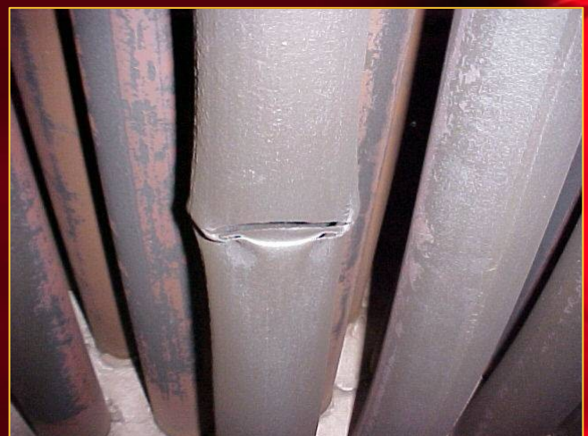
Buckled Tube with Associated Failure
