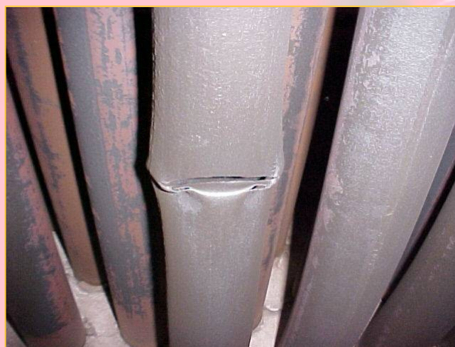
Buckled Tube with Associated Failure
