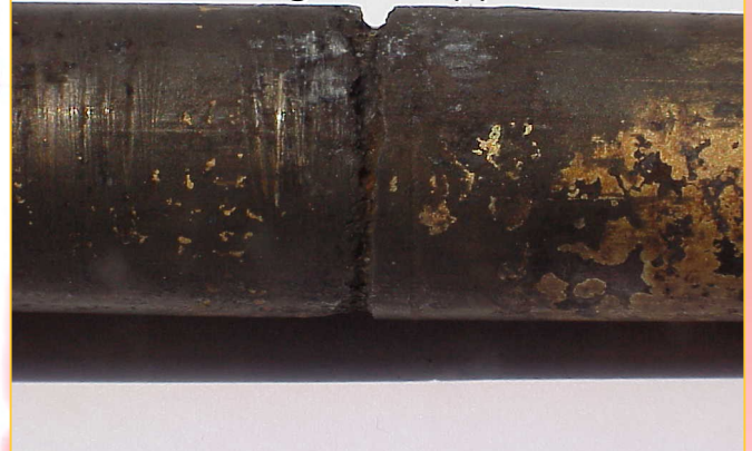
Severe groove depth adjacent to edge of support.
