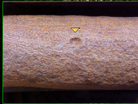
Isolated deep pitting
