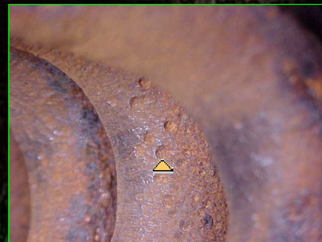
Pitting at u-bends, 40% depth
