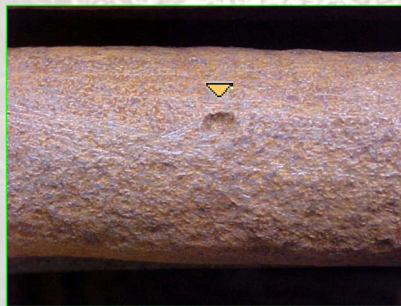
Isolated deep pitting
